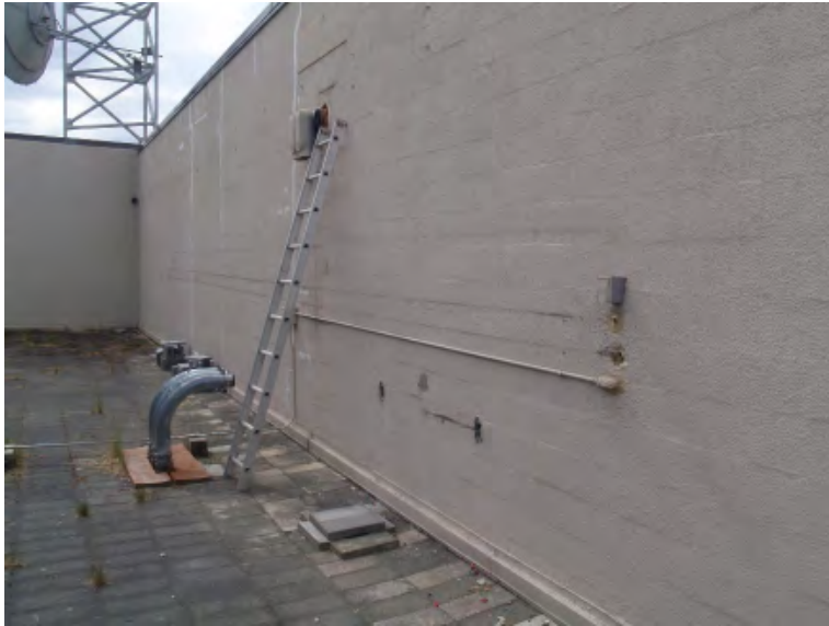
16. Roof 3 facing south. This wall is thought to be a source of wind driven leaks. Large curved roof conduits to be removed. See drawings for wall conduit treatment.
