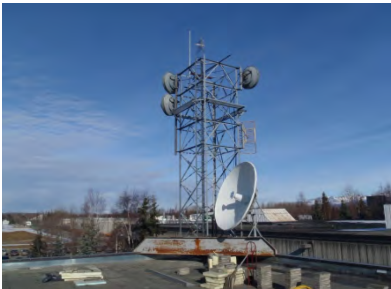
6. Antennas, support tower & base support beam at northeast corner of Roof 1, to be removed. See 1/A6.
