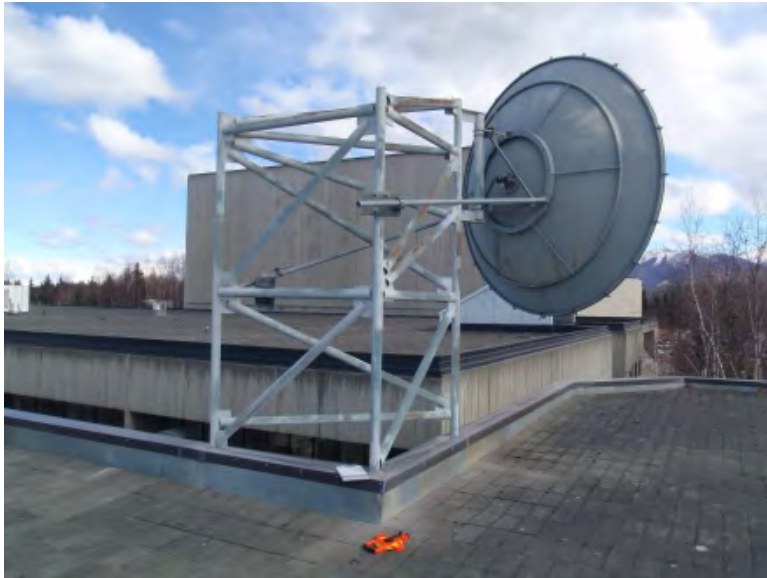
7. Antenna and support structure near south end of Roof 1, to be removed.
