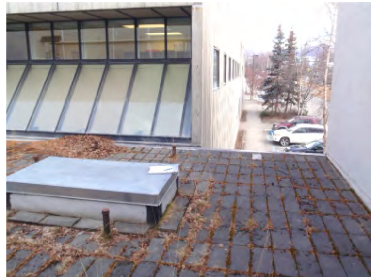
15. At south end of Roof 3 facing east. Capped curb & capped pipes to be removed.
