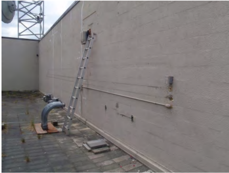
13. Low Roof 3, facing southwest. Remove existing conduit (Base Bid). New siding work on this wall (Additive Alternate #1). Install new wall conduit and j-box (Base Bid).
