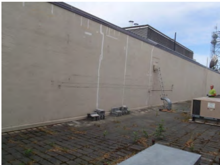
12. Low Roof 3, facing northwest. New metal siding system to be added to part of this wall (Additive Alternate #1).
