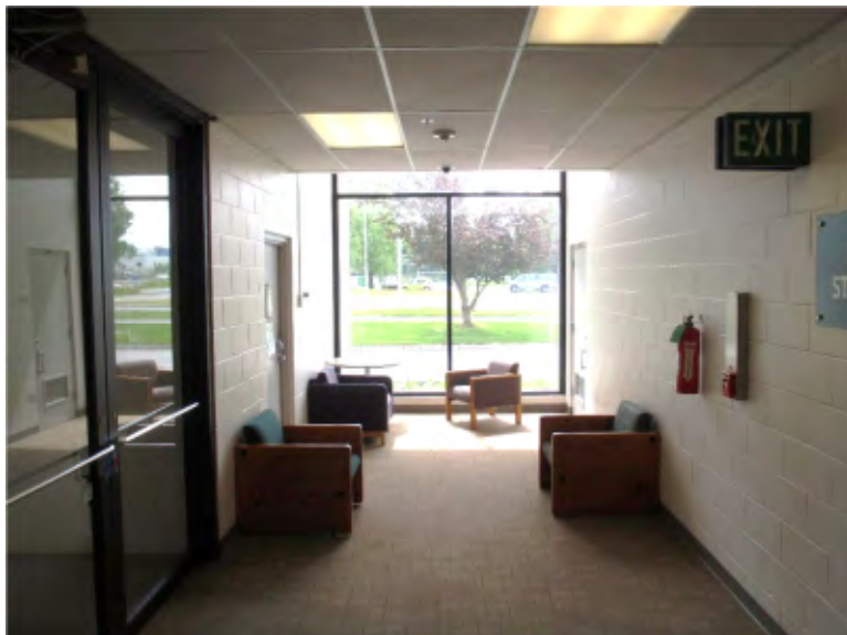
21. South end of corridor below Roof 3. Existing roof drains are above suspended ceiling next to CMU wall on right.
