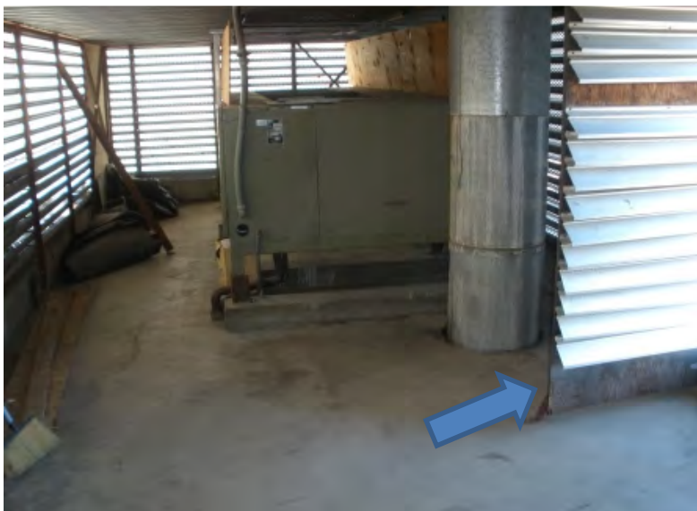
9. Penthouse interior under Roof 2, facing south. Note door (arrow) with bottom to be modified.
