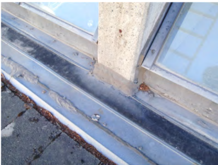
18. East edge of Roof 3 with sloped windows and building seismic joint at base. See details.
