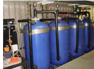
Regatta Ion Exchange tanks (ADEC photo)
