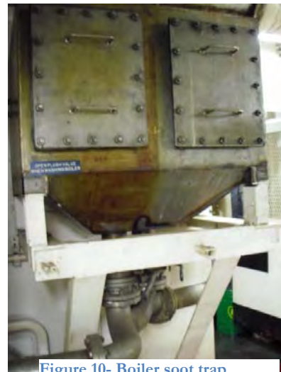
Figure 10- Boiler soot trap
