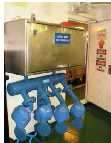
Figure 5: Potable Water Cabinet
