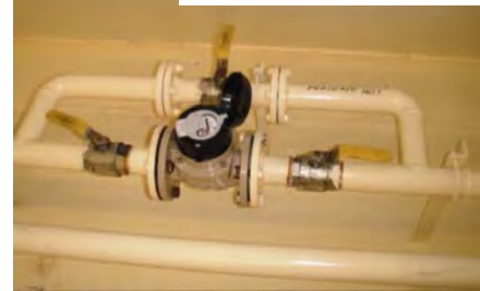
Figure 15: WW flow meters
